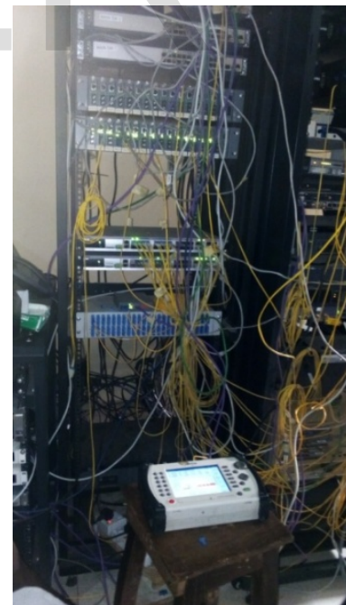
Fig. 5. Showing the connected OTDR with the patch panel or network switch at the server room while readings were being acquired
